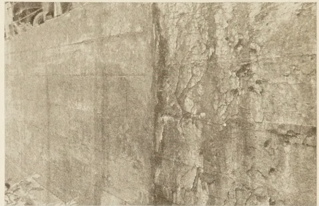
FIGURE 1.—THE LEFT HALF OF THIS CONCRETE RETAINING WALL CONTAINS SATISFACTORY AGGREGATE; THE RIGHT HALF CONTAINS UNSOUND LIMESTONE.
